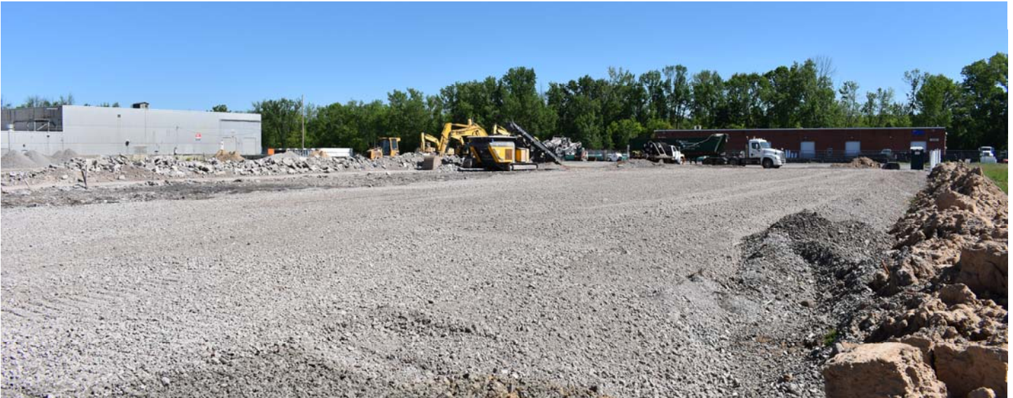
Former foundation of FRP-1 in the foreground, FRP-2 and Garage in the background
