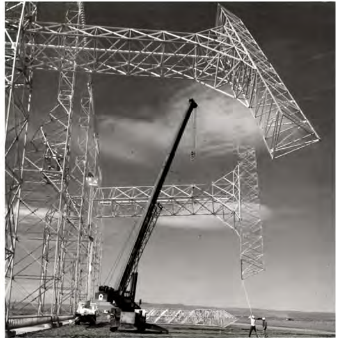
July 15, 1988 - One of the antennas for General Electric's Over-The-Horizon (OTH) Backscatter Radar system is being erected.
